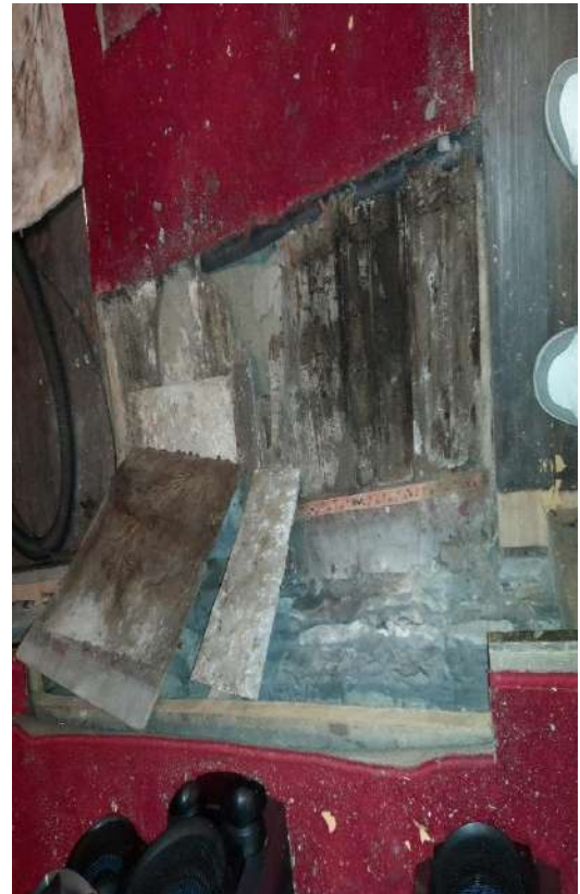
The rotten flooring left by the removal of the organ. The half-visible white trainers on the right of the photograph (owner unknown) cleverly give you a sense of scale.
